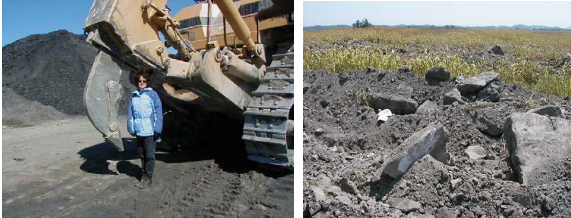
Figure 10: Deep soil ripper on large dozer and loose-graded spoil (Sweigard et al, 2007)
